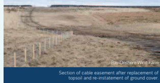
Ray Onshore Wind Farm Section of cable easement after replacement of topsoil and re-installation of ground cover.
