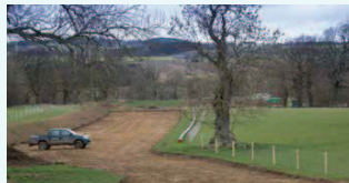
Ray Onshore Wind Farm Section of cable easement with topsoil stripped prior to trenching operations. Note: topsoils storage mound (on left) ensures soil quality is preserved. Temporary fencing delineates working area.
